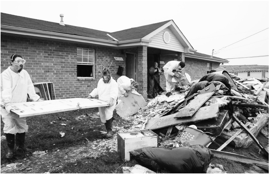
Volunteers with Common Ground help clean up the toxic aftermath of Hurricane Katrina, 2005.
