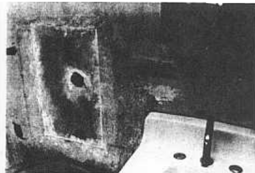
DEADLY LEAD POISONED WASHROOM WALLS
