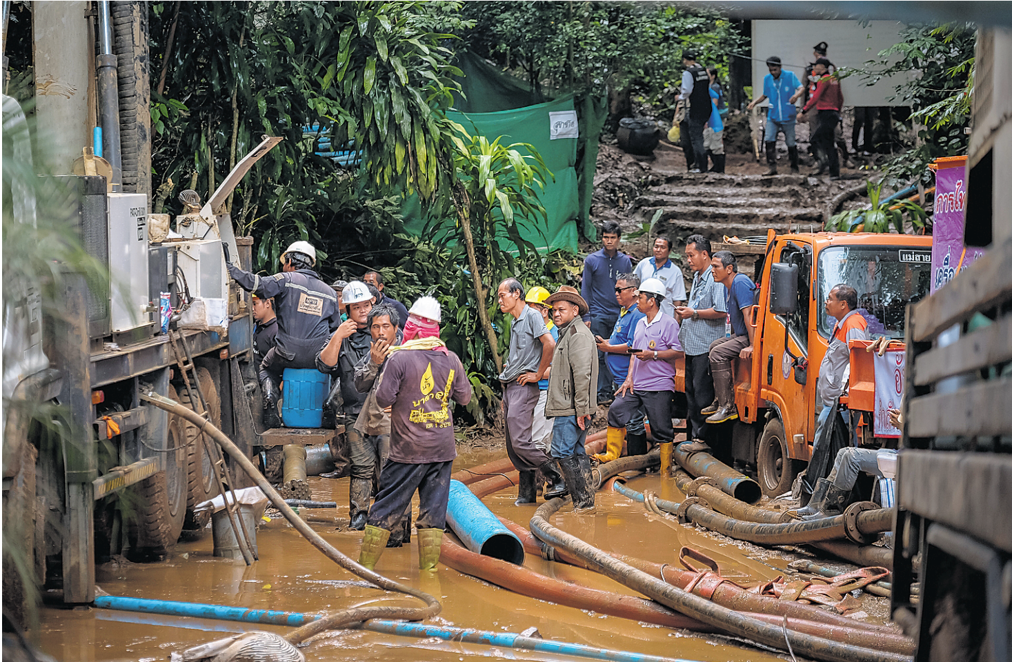
Rescue workers used a water-pumping machine at the entrance to the Tham Luang cave complex in northern Thailand on Monday.
