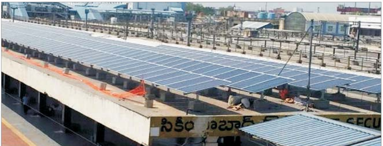
500 kWp grid connected Solar rooftop power Plant at Secunderabad Station
