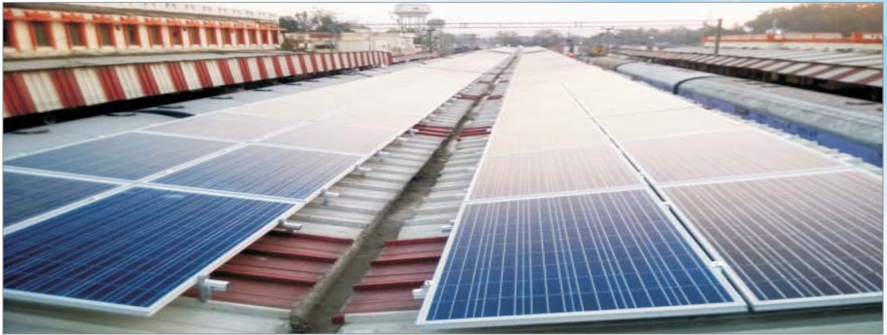
500 kWp Solar rooftop power plant at Varanasi Railway Station
