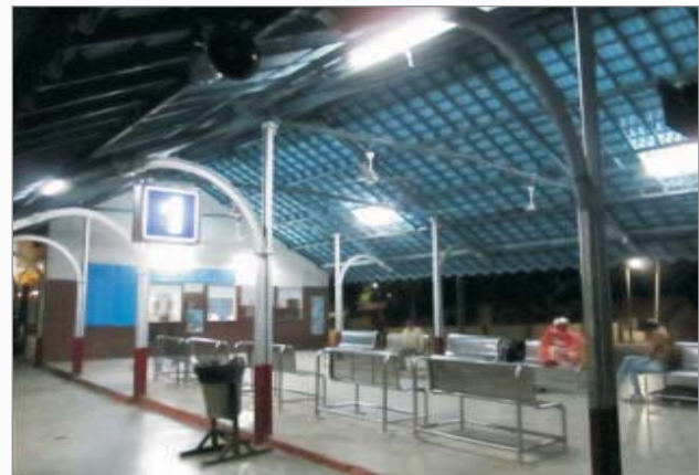
LED lights installed at Railway stations
