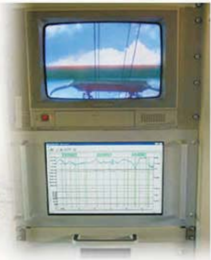
Tower Car with Measuring & Recording Instrumentation (for predictive maintenance)
