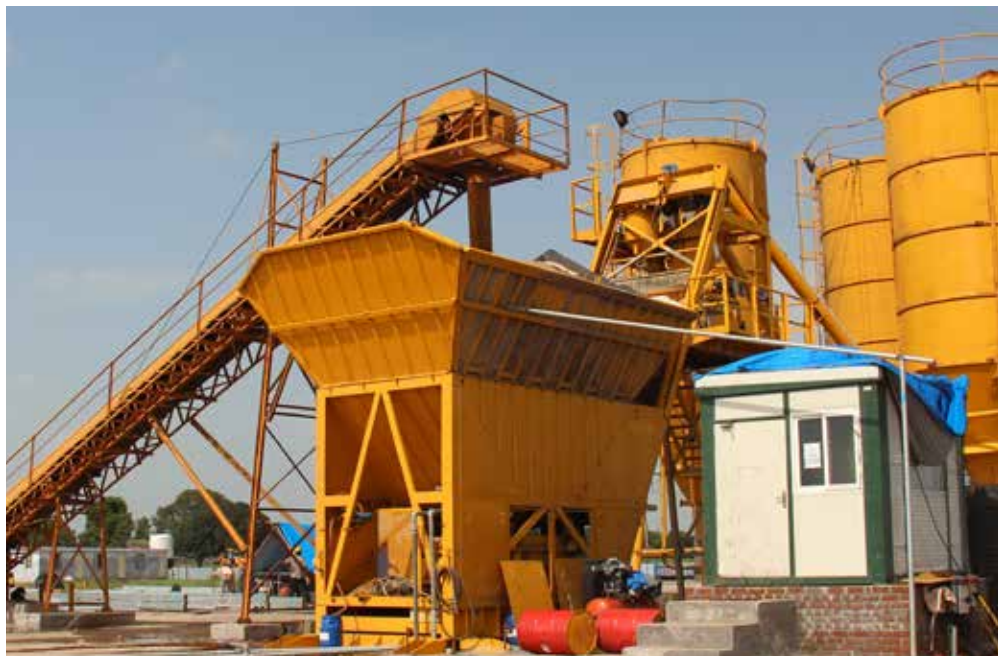
Figure 25. Concrete batch mix plant.
