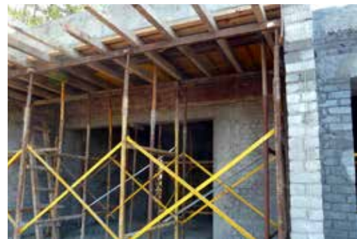
b) Slab formwork was supported with steel props during and after construction
