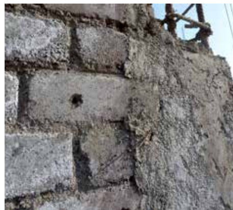
c) Masonry wall surface showing a hole in a brick created to secure the formwork in place
