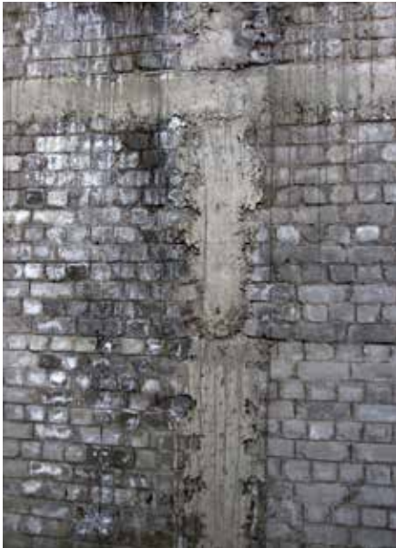
a) An interior tie-column after construction (note the construction joint at the wall mid-height)
