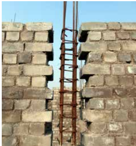
a) Tothed wall edges at an interior tie-column
