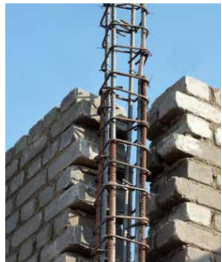
Figure 11. Tothing at the wall-to-tie-column interface.
