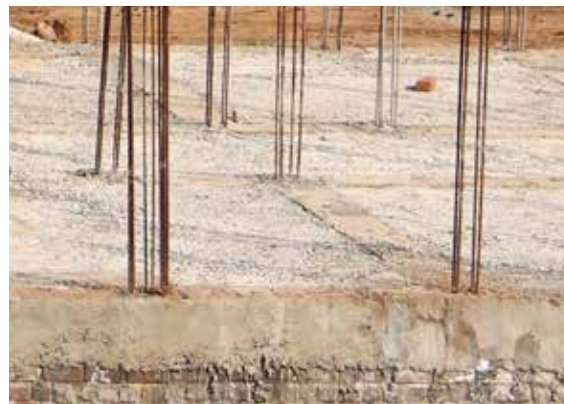
Plinth level in a building showing tie-column reinforcement extending above the plinth band
