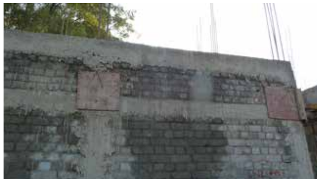
Figure 45. Confined masonry wall under construction - note a completed RC lintel band and RC tie-beam at the floor level and formwork for tie-columns above the lintel band.
