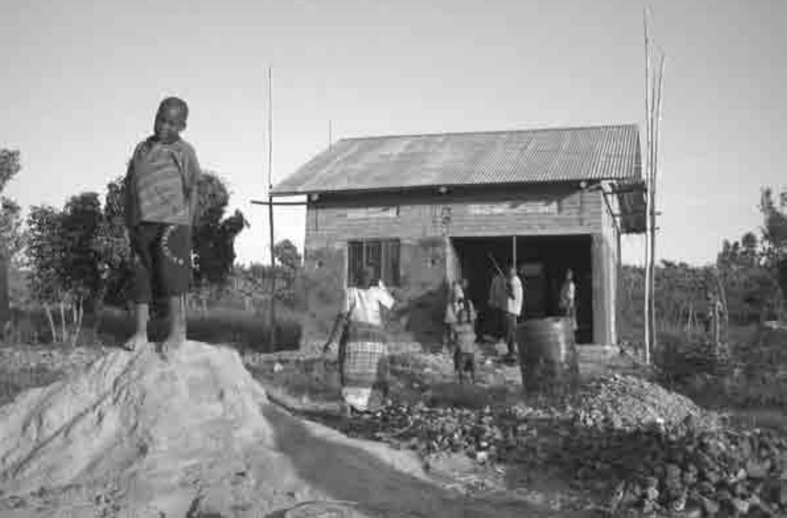
Katuulo organic farming community in Uganda, construction of a health centre which has since been completed. Photo by Kristen Lyons.
