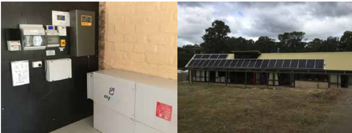
Figure 23: Jayne and Cathy's house with solar panels, inverter and battery system (Source: Jayne and Cathy)
