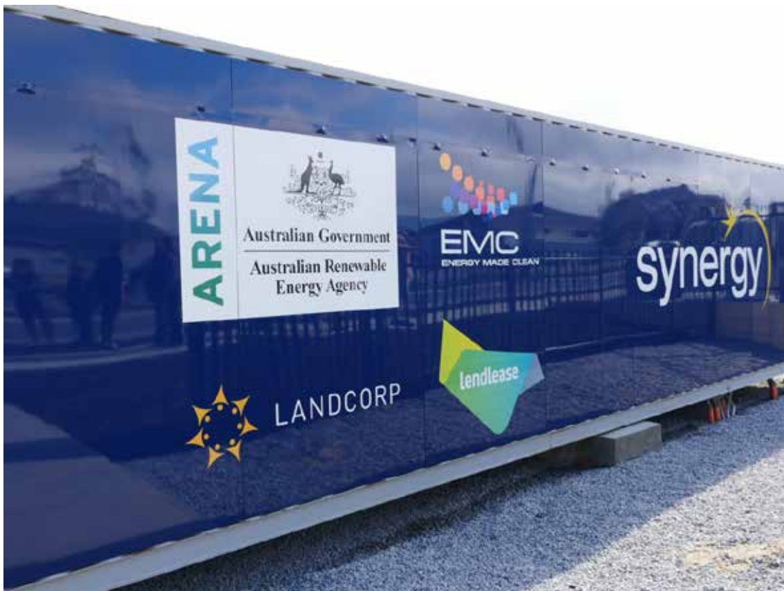
Figure 24: Alkimos community storage battery container (Source: Synergy)
