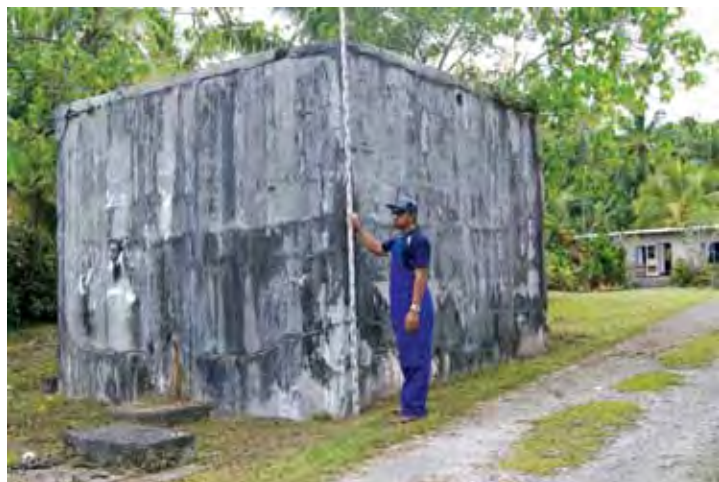
Old infrastructure, such as this water tank on Niue which dates from the 1960s, contributes to vulnerability of communities.
