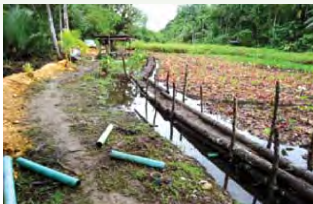
Dikes are helping to reduce saltwater intrusion in the trial sites.
