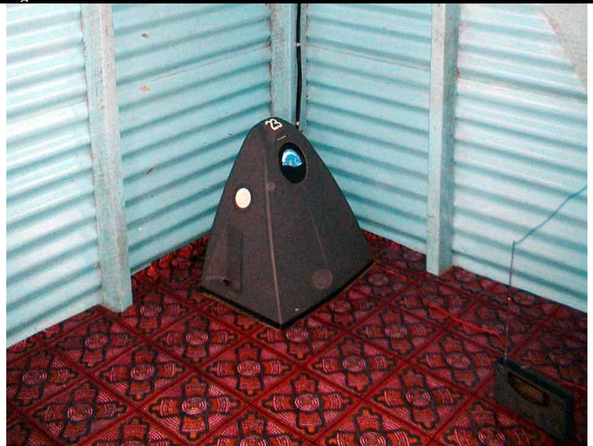
Fig 5-20. The Shell Powerhouse installed in a Vunivau house
