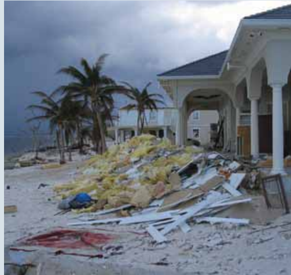
Impacts of Hurricane Ivan on coasts not protected by the reef in Grand Cayman
