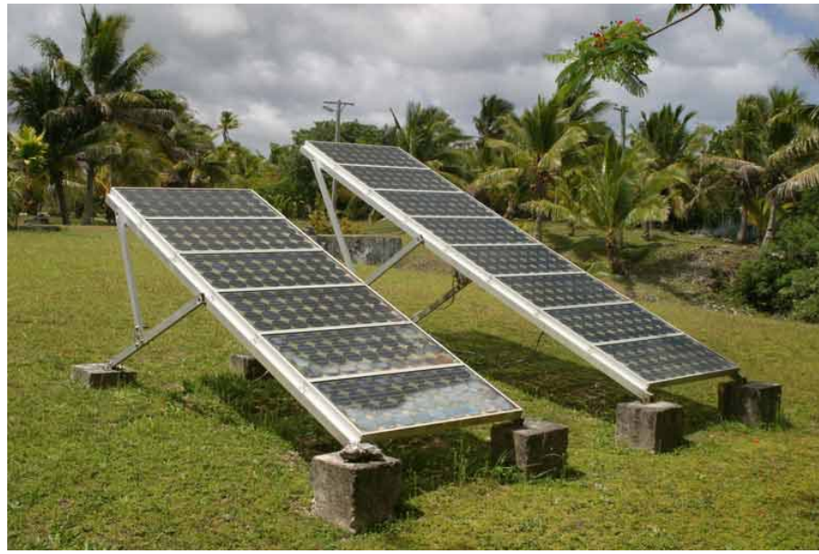
Figure 4-13 – Solar PV Panel, Namukulu Community Hall, Niue
