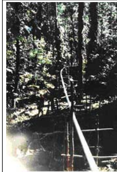
Figure 3-4 – Irii Hydro Penstock, Solomon Islands
