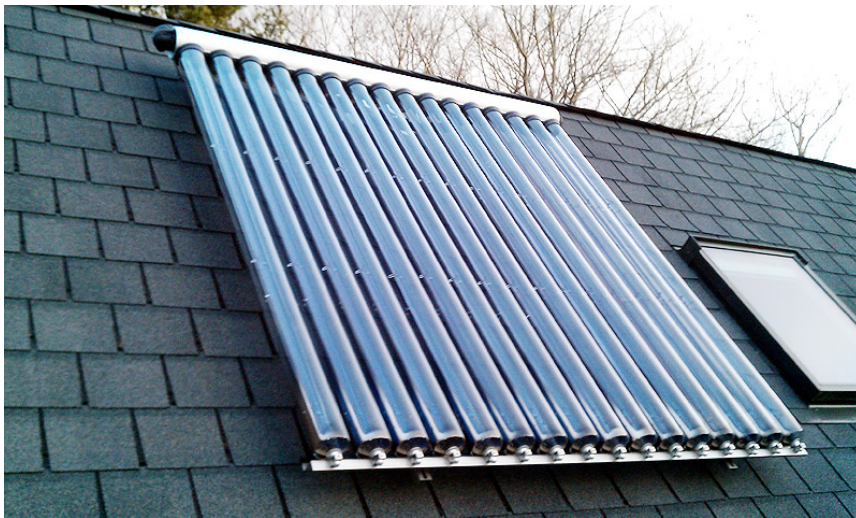
Figure 2.4: A rooftop solar thermal array for domestic water heating.
