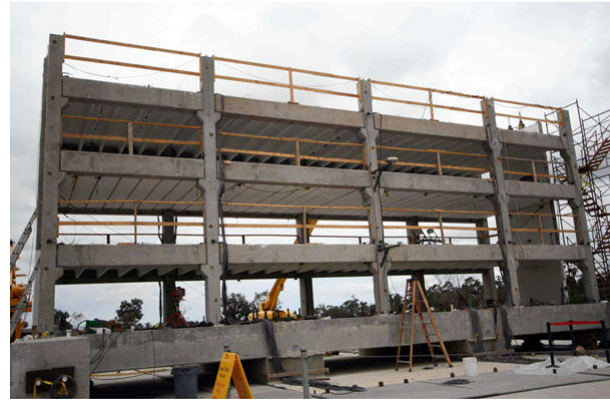
Figure 8. Test of a half-scale model of a three-story parking garage on the shake table at the University of California (UC) San Diego’s Englekirk Structural Engineering Center. The UC San Diego shake table is an element of the NEES infrastructure, the largest shake table in the United States, and the only outdoor shake table in the world. This study is supported by NSF, NEESinc, the Precast/Prestressed Concrete Institute, and the Charles Pankow Foundation. © 2008 by UC San Diego Jacobs School of Engineering.
