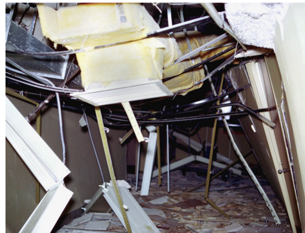
Figure 11. Nonstructural damage (fallen ceiling, partitions, piping, and ducts) to the basement of the Olive View Medical Treatment Building caused by the 1971 San Fernando earthquake in California. © 1971 by Earthquake Engineering Research Center and Regents of the University of California.
