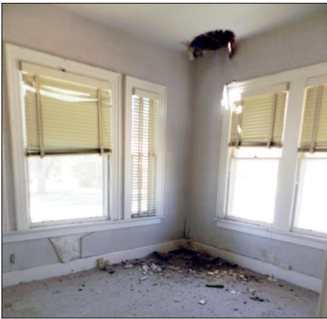
Interior damage of Kerrville Medical Center.
