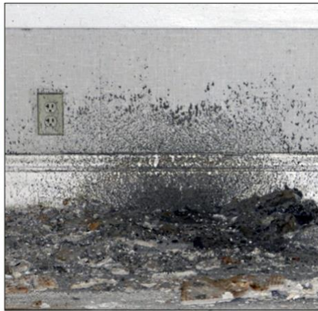
Portions of the ceiling have collapsed, spraying debris on to the floors and walls.
