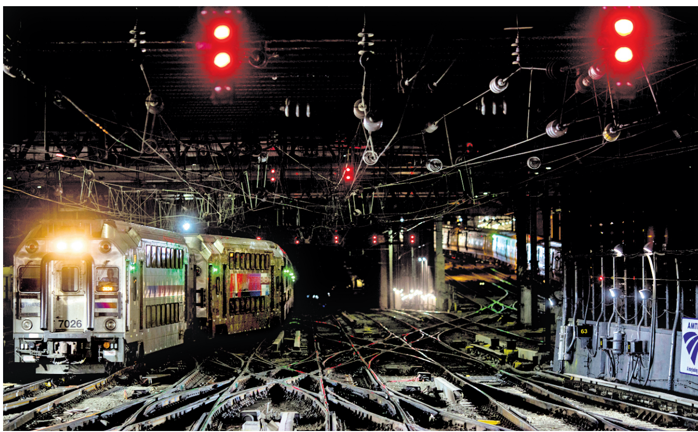
Interlocking A, a tangled sorting mechanism that routes trains entering and exiting Pennsylvania Station in New York.
