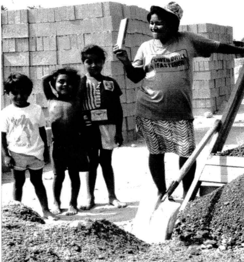
In an impoverished shantytown community in San Salvador, families are building their own homes as part of a collective construction project.
