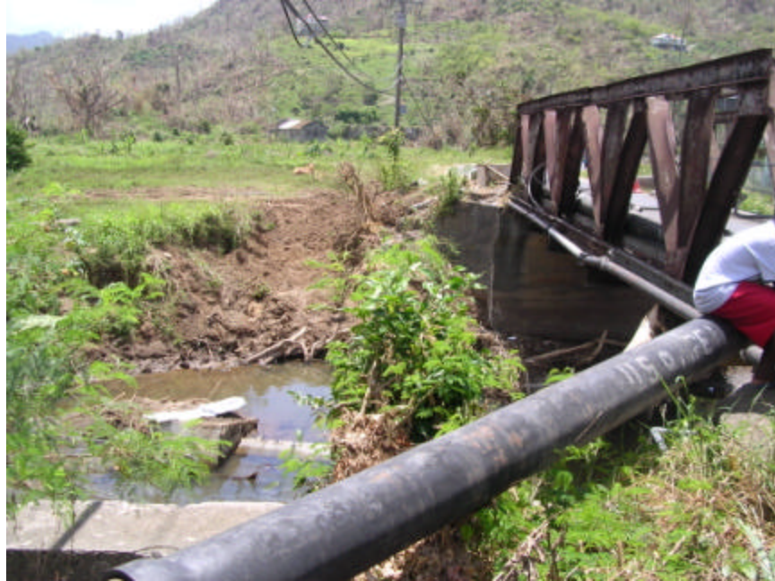
Photo 6 Damaged Water Supply Infrastructure at Beausejour
