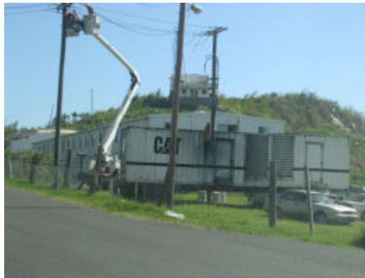
Photo 5 1.5 MW Unit in Lance Aux Epines
