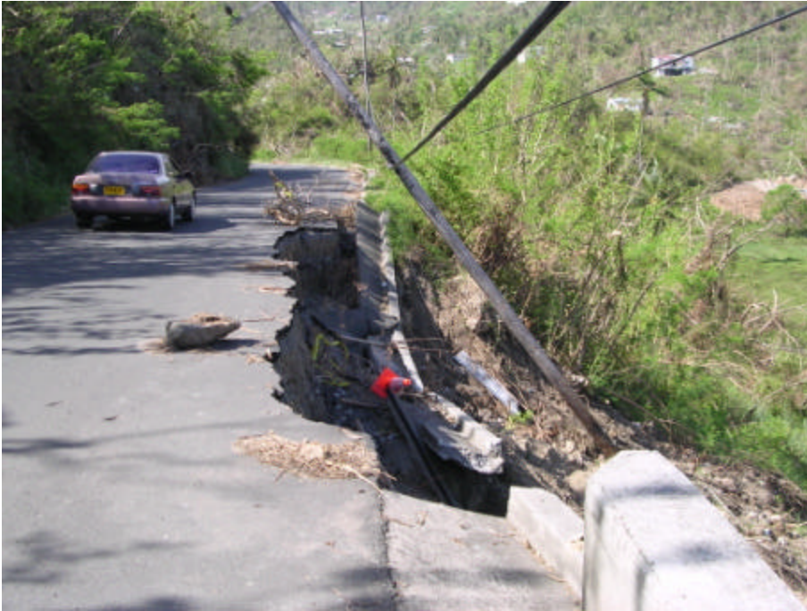
Photo 9 Erosion of Roadway at Westerhaul
