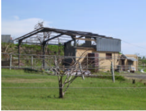
Photo 12 Total Collapse of Walls of Store Equipment Building for PSIA
