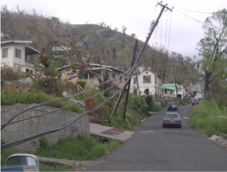
Photo 7 Downed Poles Carrying Communication Cables
