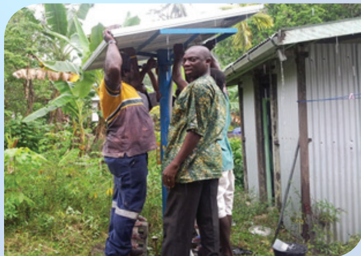
UNV EPI Officer Robert Ninson and staff of the National Medical Stores, together with health staff of Lambi Clinic and community volunteers, help in installing a solar panel.
