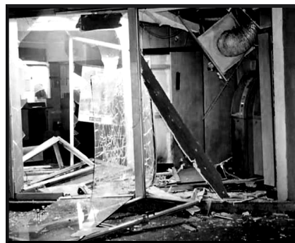
Remains of a banking institution in Mexico City after an explosive attack by 'Autonomous Cells of the Immediate Revolution' - Praxedis G. Guerrero', 03.10.11
