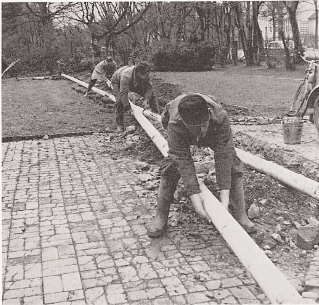
At the beginning of 1961, for the Yves Klein exhibition in Krefeld which opened on 14 January, the workers install gas pipes in the Museum gardens...
