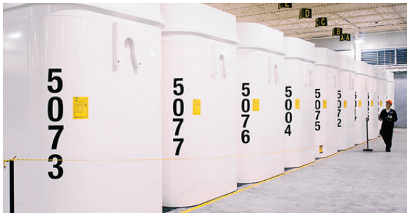
USED FUEL STORAGE CONTAINERS
