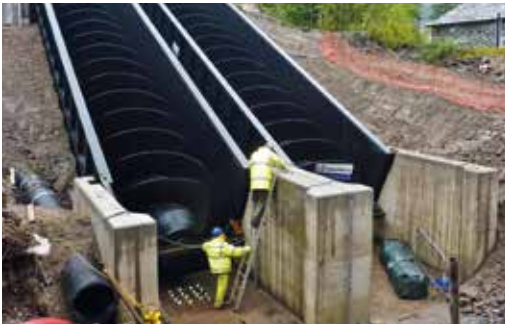
FIGURE 4.7 A hydro-electric installation at Low Wood, Haverthwaite
