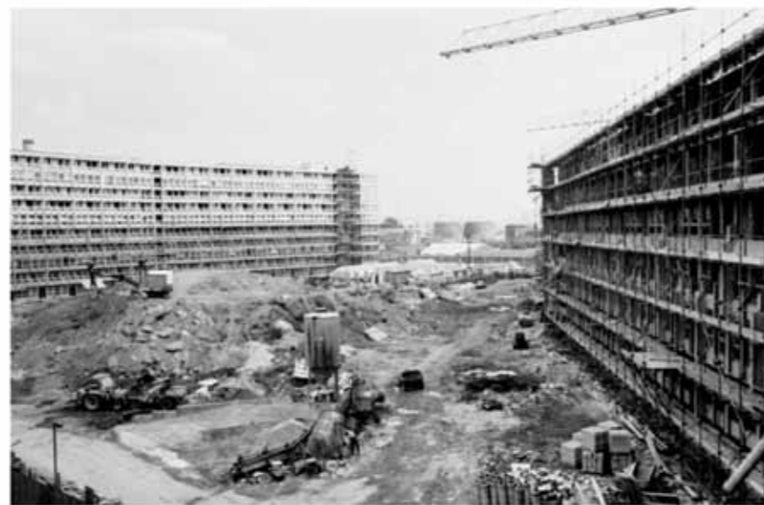
Fig. 8.5 Piles of debris in the Robin Hood Gardens, by Alison and Robert Smithson, 1970
