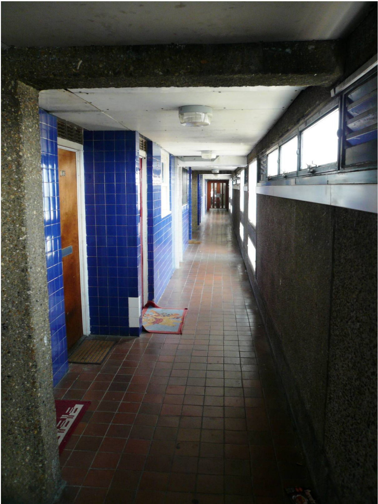
Figure 3: Indefensible spaces? Interior walkways between lift shaft and flats in the Balfour Tower. Photograph taken in 2008 by Rodney Harrison.
