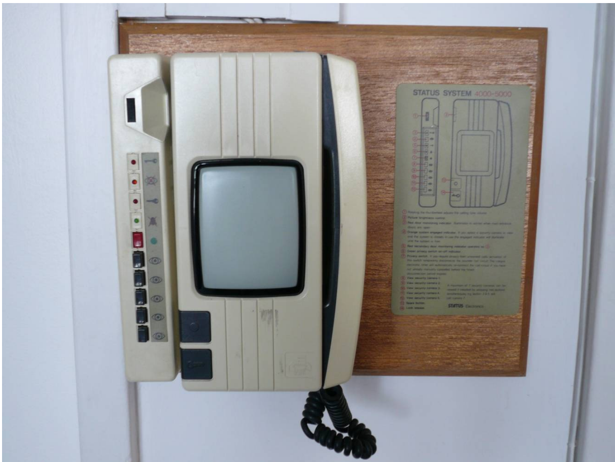
Figure 4: ‘Seeing like a state’: Surveillance camera entrance phone, installed during the late 1980s or early 1990s inside Balfour Tower flats. Photograph taken in 2008 by Rodney Harrison.
