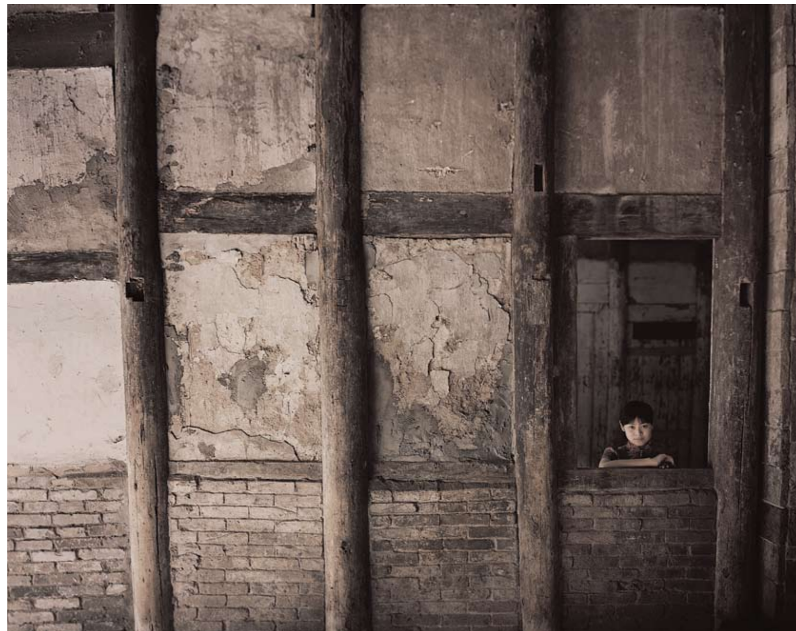
THIRD FRONT — OLD WALL 2004
