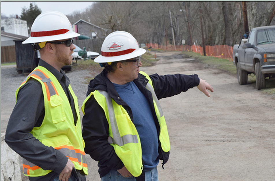
Matt McKissick, project engineer, and Bob Tramontina, construction control representative, oversee the more than $880,000 shoreline reclamation project.
