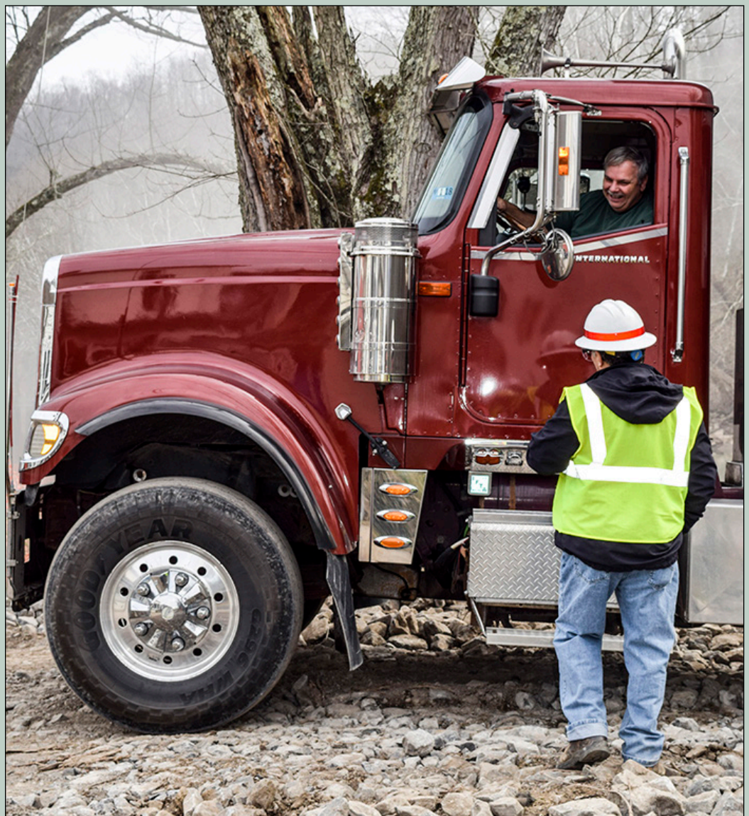
Bob Tramontina, construction control representative, Pittsburgh District, talks with a riprap dunk-truck driver working to protect a sanitary sewer line that runs along the West Fork River bank.
