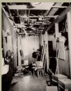
Bomb damage at CIS (1971).
