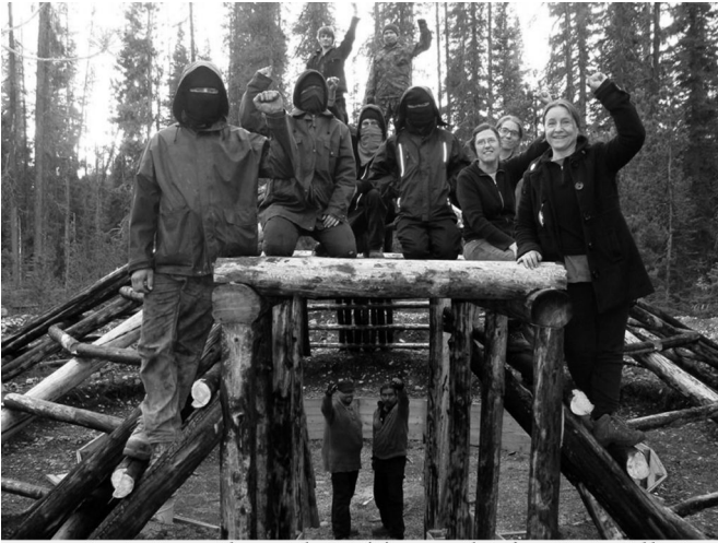
Constructing a pit house at the Unistoten camp. Photo from Warrior Publications.
