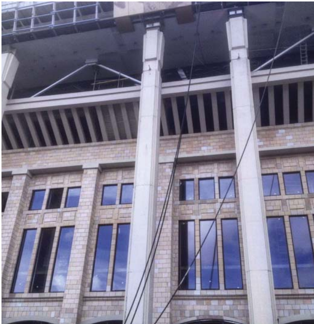
Ceramic tiles on the historic outer envelope of Luzhniki Stadium are being restored and missing tiles replaced with new ones manufactured in the same way as the original items.
