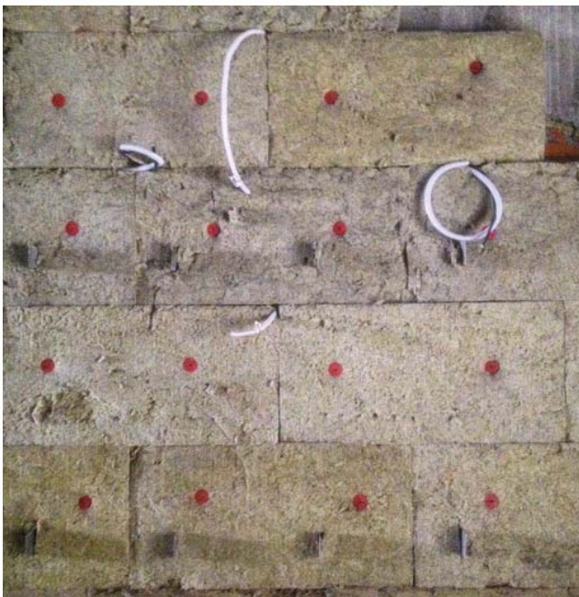
The thermal insulation of the walls is based on material manufactured by a specialised company in Russia.
