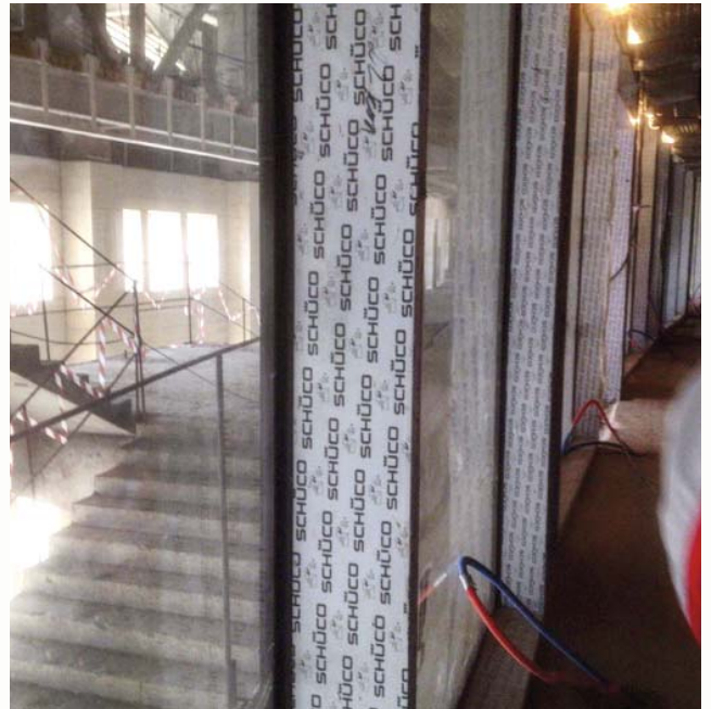
Window openings are filled with AGC glazing systems based on argon-filled double-pane units. The glazing units are fitted into Schüco aluminium profiles, which are considered to represent the best quality available on the market.
