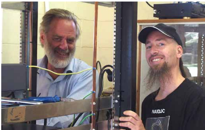
3CR technician Riah with Wayne Dickson of Commercial Radio Australia installing a digital repeater at the Werribee transmitter site
