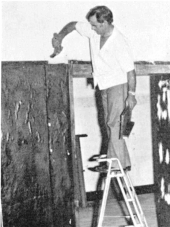
Mr Doug Scott busy in January doing one of the many jobs required to renovate the Aboriginal Arts and Crafts shop at the Foundation for Aboriginal Affairs
