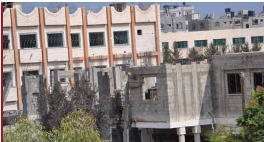
Destruction of offices of the Physically Disabled Persons` Association in al-Zaitoun neighborhood in the southeast of Gaza City
