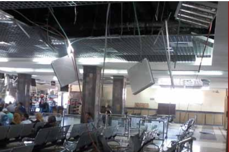
Destruction in Rafah Crossing hall
