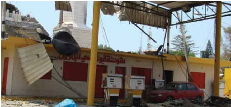
Traces of damage in Abu Assi gas station due to an Israeli attack on the neighboring mosque in al-Wehda Street in Gaza City
