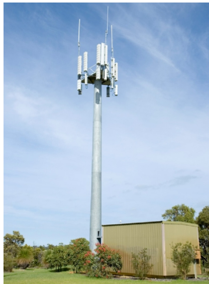
Figure 11 Base station tower
