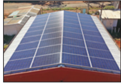
The solar system at Kurrawang.
