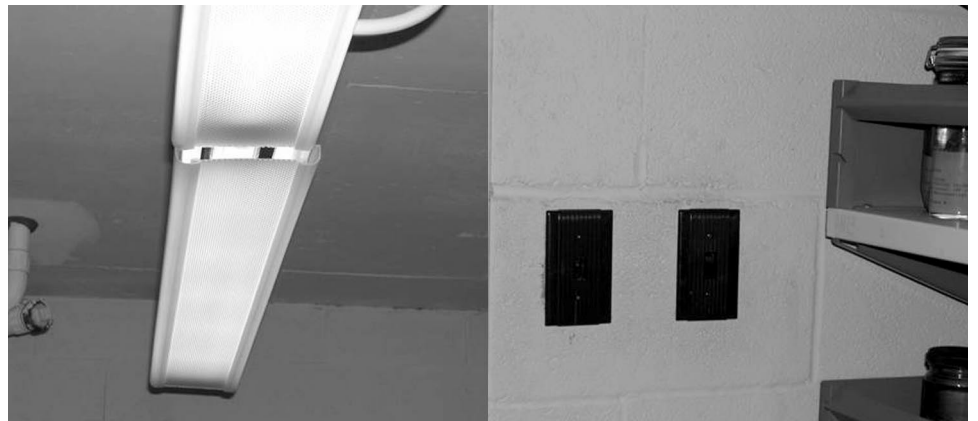
Figure 10: Nonexplosion Proof Lighting Fixtures and Switches in Alcohol Storage Rooms at the National Museum of Natural History
