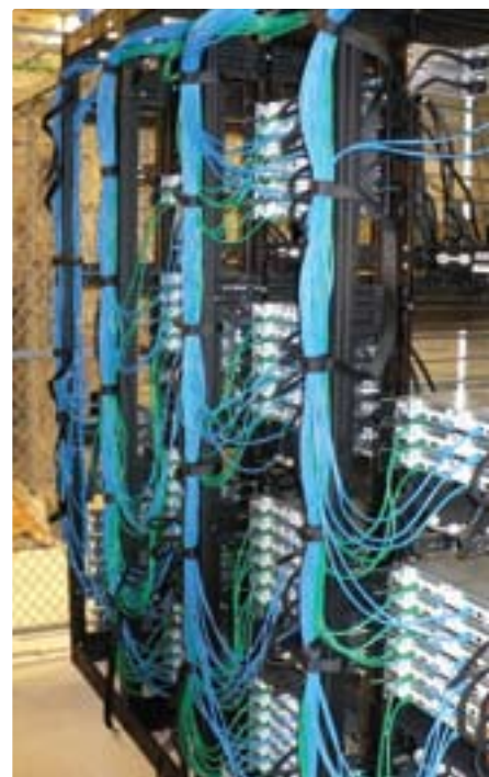
Tampa data center
