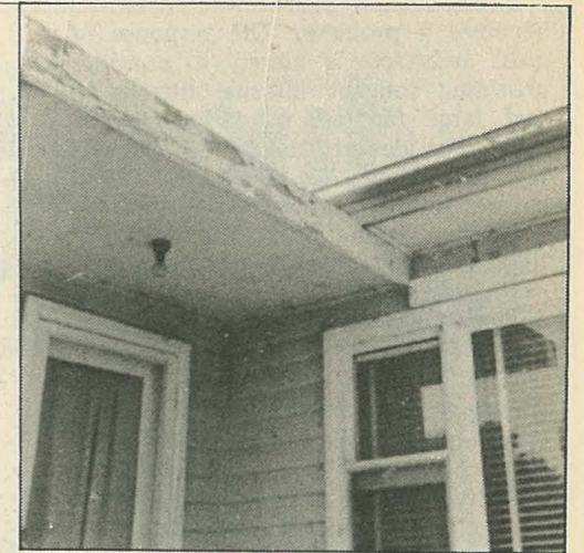
Above: Waiting time for repairs on Ministry of Housing homes is long.
