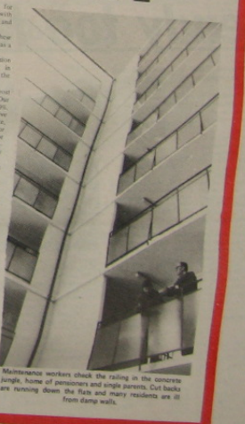
Maintenance workers catch the falling in the concrete are running down the flats and many residents are ill from damp walls.
