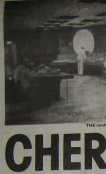
The control room at Chernobyl.
