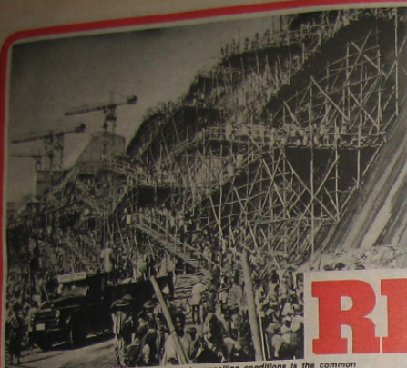
MASSIVE NUMBERS of workers labouring under appalling conditions is the common impression that must unite India's burgeoning working class. Above, dam workers on the River Krishna.
