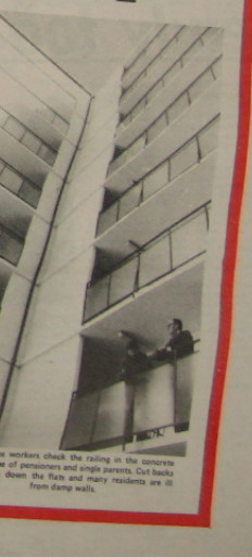
Maintenance workers catch the falling in the concrete are running down the flats and many residents are ill from damp walls.
