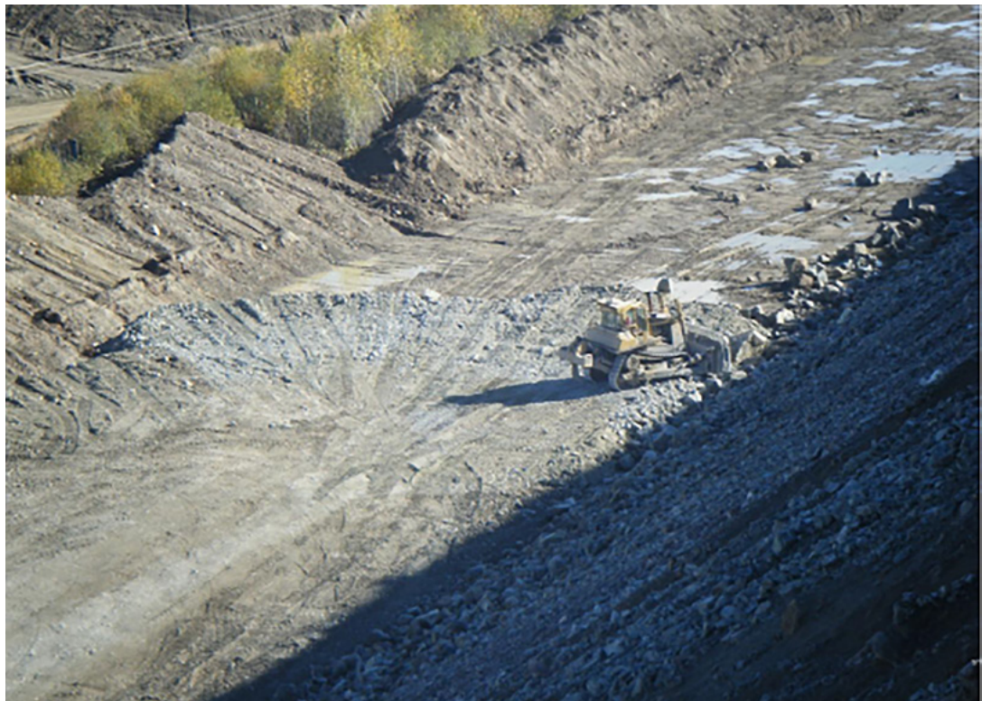
Figure 6.23 C Zone Material Placed in PE Subexcavation, October 19, 2013 AMEC Environment and Infrastructure (2013b)
