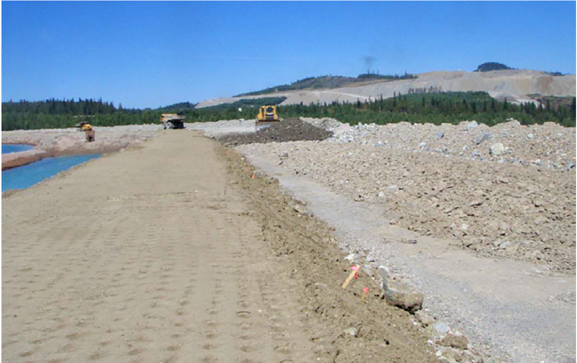
Figure 8.2 Placement of Zone C Rock on PE, July 28, 2014 AMEC Environment and Infrastructure (2014e)
