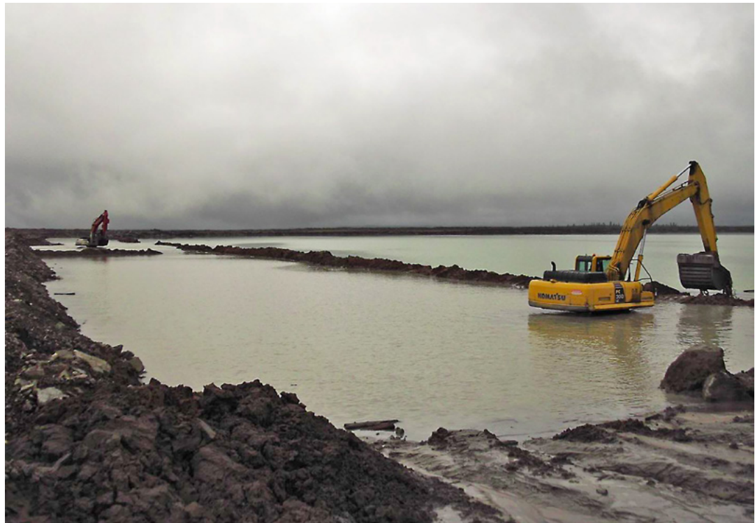
Figure 6.24 Creation of sand cells 3+150 to 3+050, on May 18, 2014, indicating high water level 6 days before the overtopping event AMEC Environment and Infrastructure (2014c)
