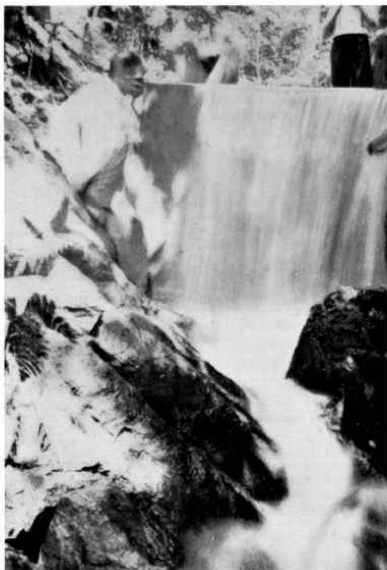
Intake Tank, Settlement Water Supply.
