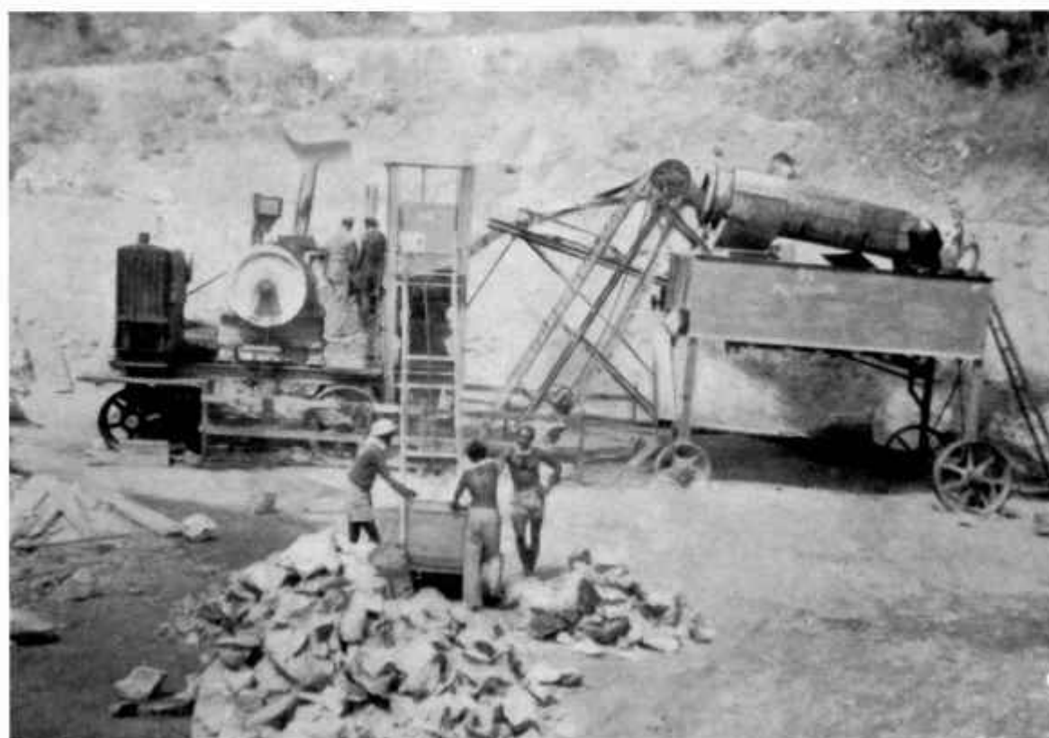
Stone Crushing Plant, Settlement Water Supply.
