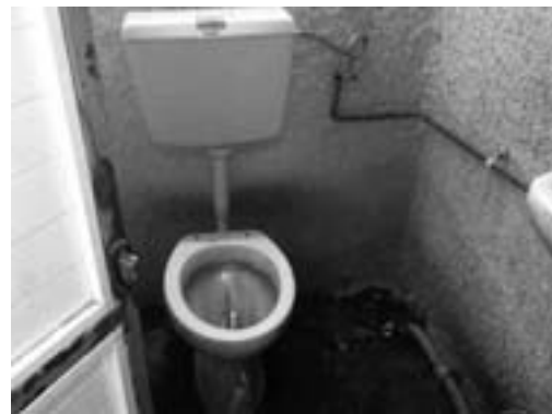
Detention centre Lesbos: At the time of our visit one functioning toilet was provided for 50 detainees.
