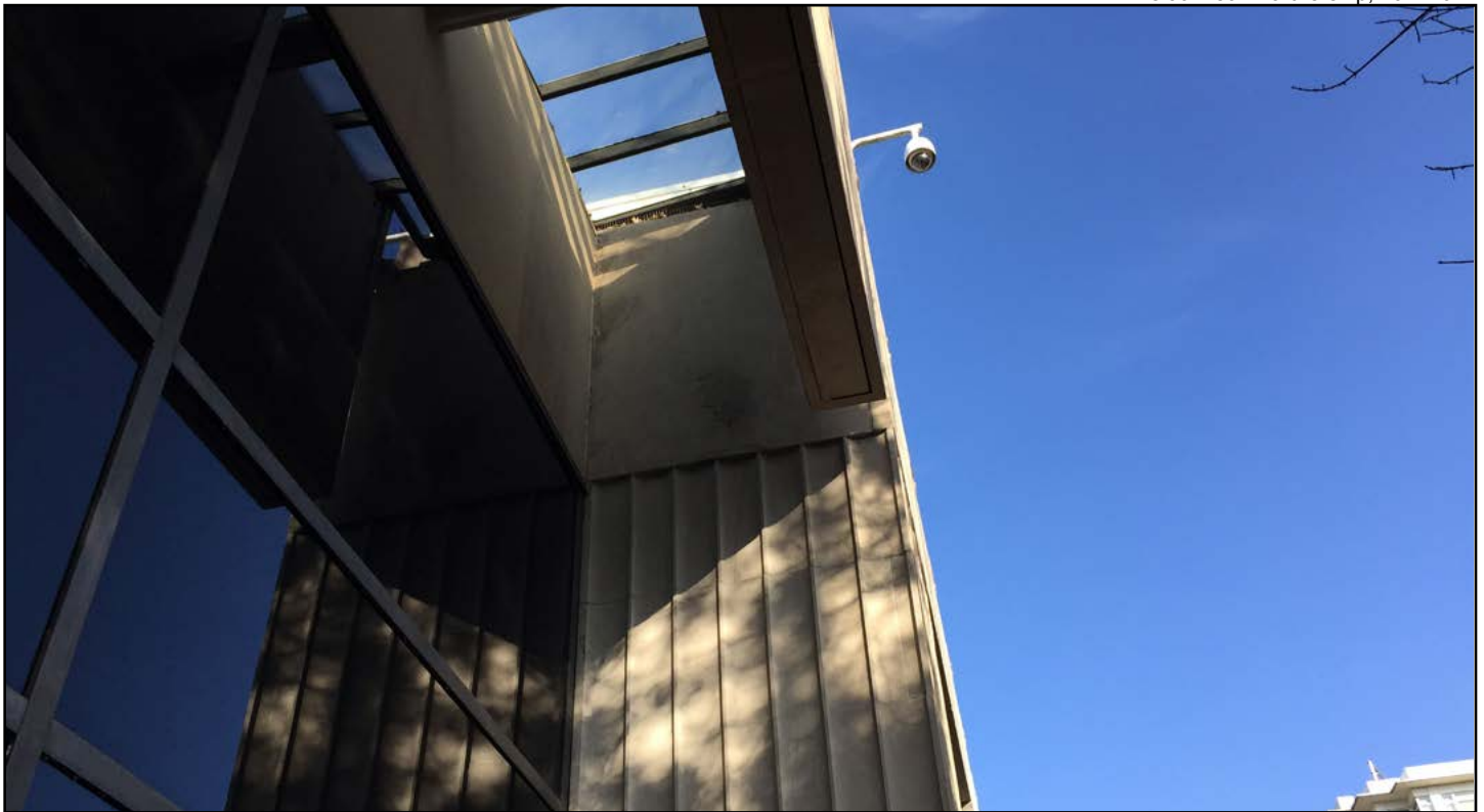
Figure 14 • Seattle Times Building Complex, detail of 1947 Office Building Addition adjoining 1979 Office Addition
