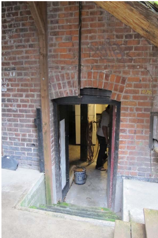
Fig. 89 – Former laundry/storage structure along alley, showing first floor entrance to mechanical room.
