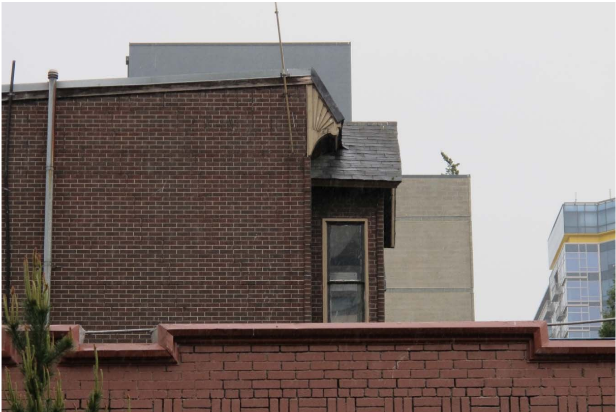
Fig. 62 – North elevation, in distance, showing remaining architectural detail at parapet.
