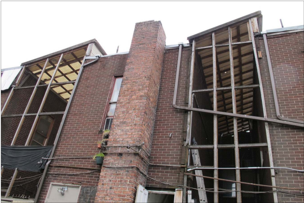
Fig. 92 – Rear deck at second floor, view of upper part of second and third floor east elevation.
