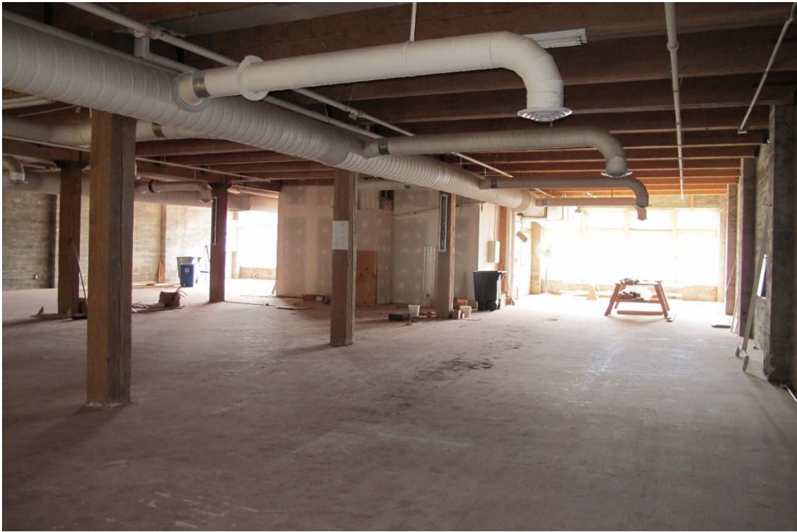
Fig. 76 – Interior, typical shell of office space, between demising walls, facing towards exterior windows.
