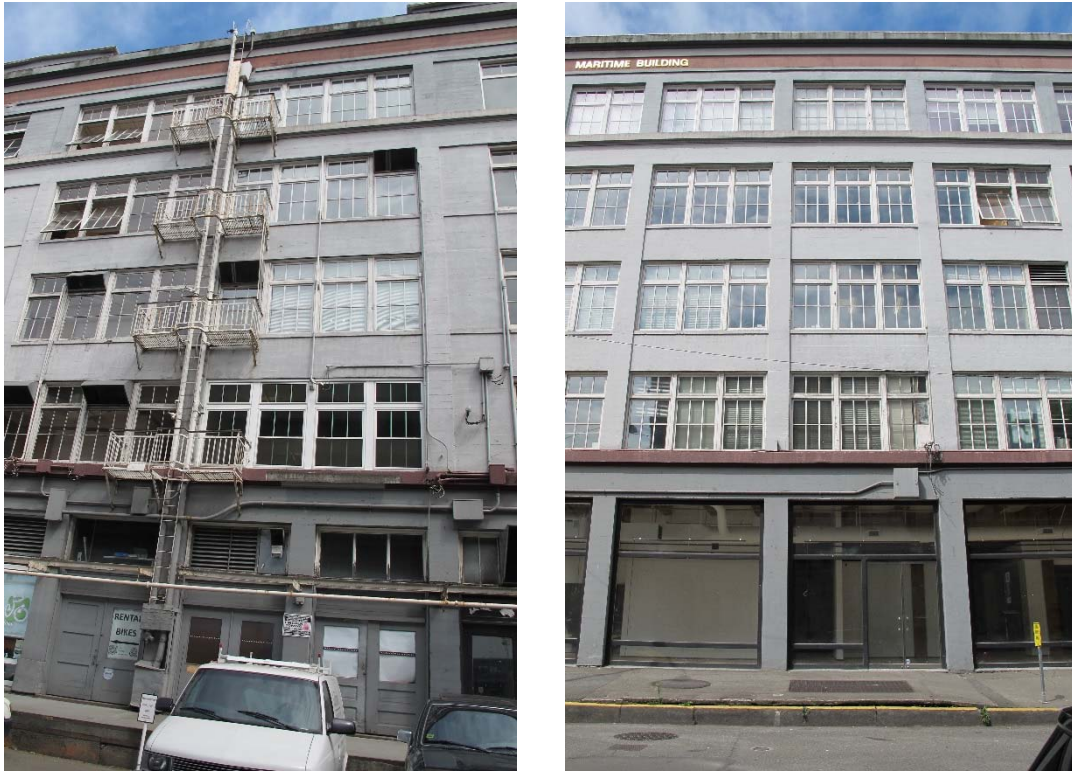
Fig. 62 – Detail, west or Alaskan Way elevation (left) and south or Marion Street elevation (right). At left image, lower right window may be vinyl sash.
