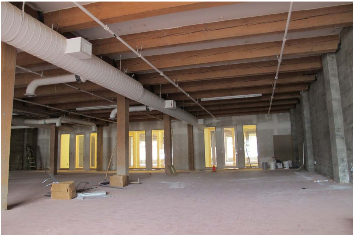
Fig. 77 – Interior, typical shell of office space, between demising walls, facing towards interior corridor.
