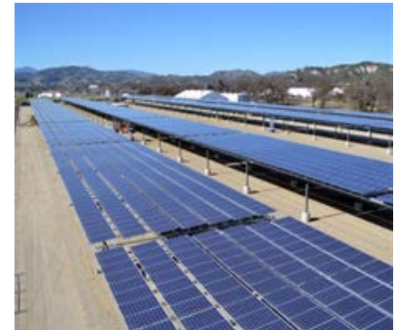
Fort Hunter Liggett 2MW photovoltaic system installed
