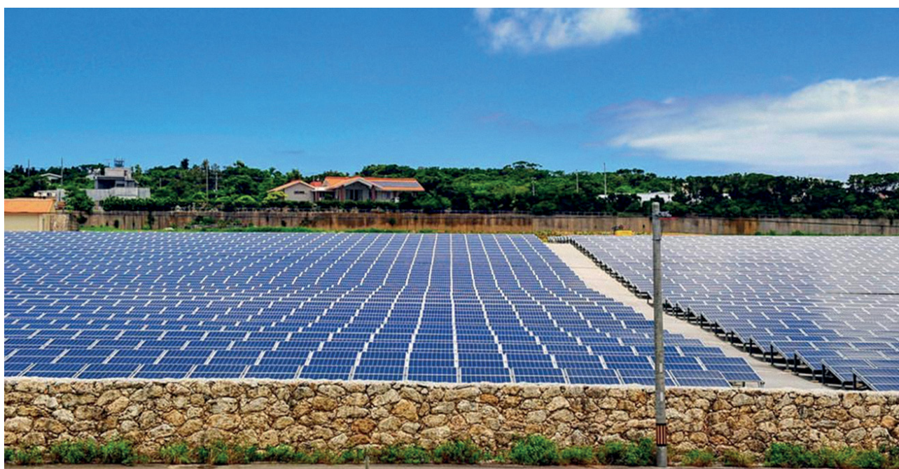
Figure 3: Solar plant in Okinawa, Japan.
