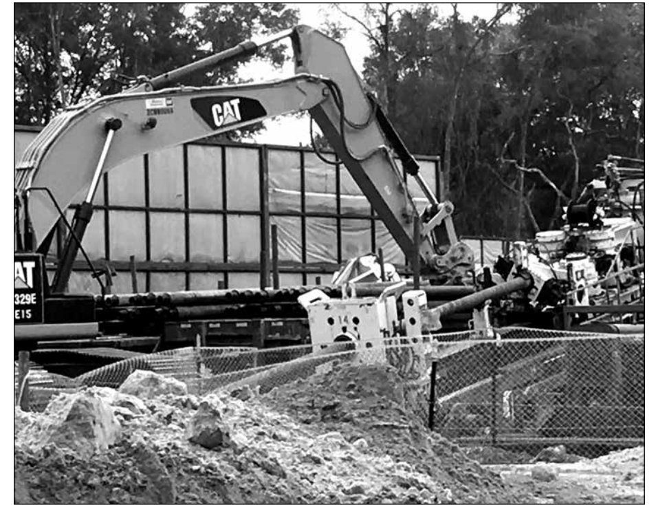
The massive HDD drill digs through the land below the wetlands and river in preparation for the Sabal Trail pipeline. Photo by Peter Ackerman.
